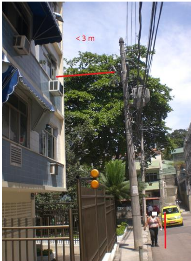
Figure 3: An IEC 60282-2 expulsion type fuse installed very near a residential window where children could be
